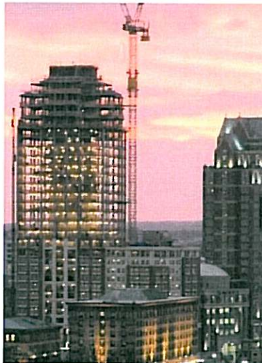
PHOTO COURTESY THE PROCACCIANTI GROUP TONIGHT in Providence, TPG will host a downcity celebration of the topping-off of the new Westin tower, complete with fireworks.
